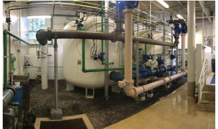
Existing Greensand Filters at Phillips Road (Constructed in 2013)
